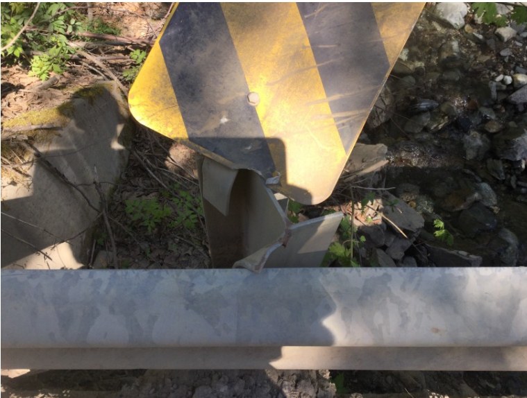
Upstream right approach riser damage
