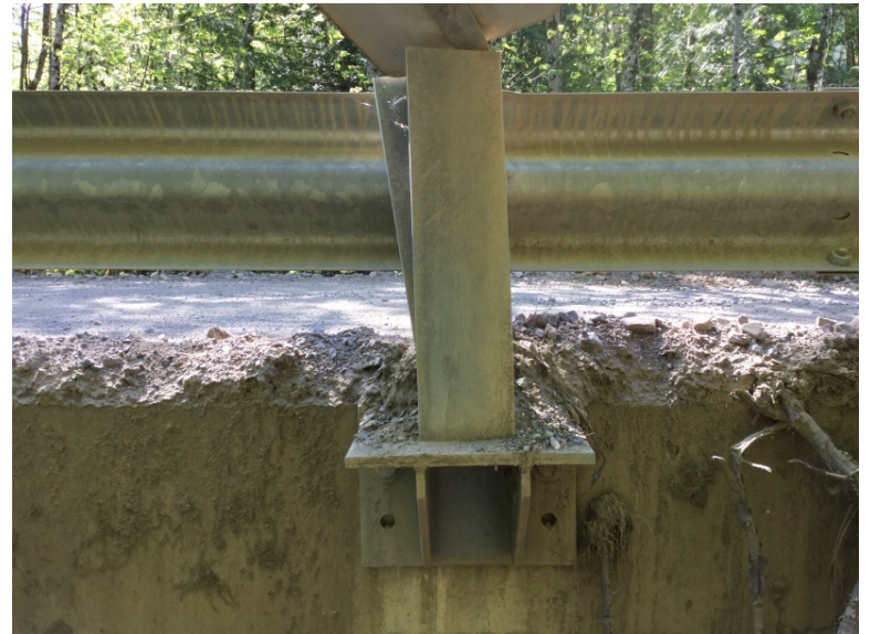
Upstream right approach riser damage
